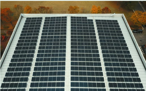
Solar power facilities at the LOTTE Chemical R&D Center
